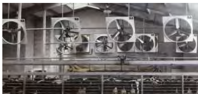
FIG. 9. Circulation fans and sprinklers over holding area.
