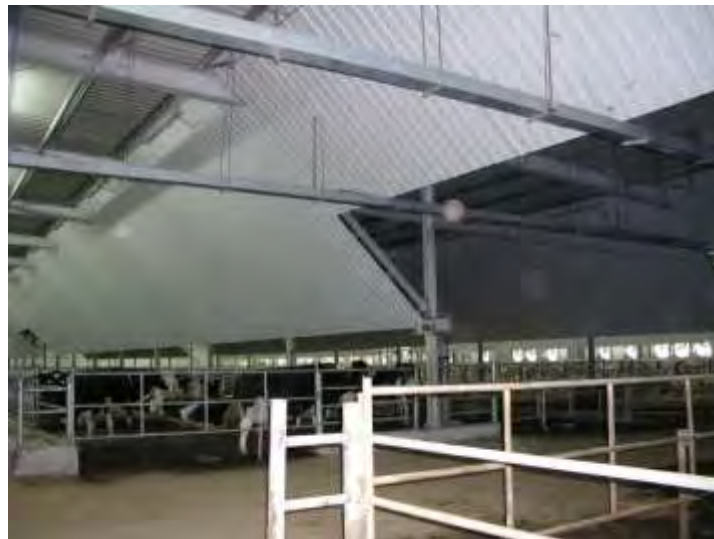
FIG. 6. Slanted baffle in cross-ventilated barn. Higher air velocity is often observed in cross alleys where baffles are higher to allow equipment to pass underneath.
